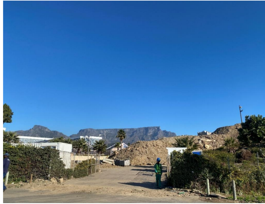
Photograph 3-8: View of the construction spoil area on site (location of the previous The Lookout Venue)
