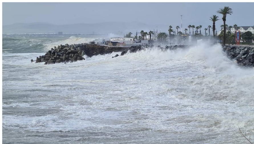
Photograph 4-4: Overtopping of rock revetment at approximately 15:00 on 13 July 2020. Photo credit: Stephen Luger (PRDW, 2023)
